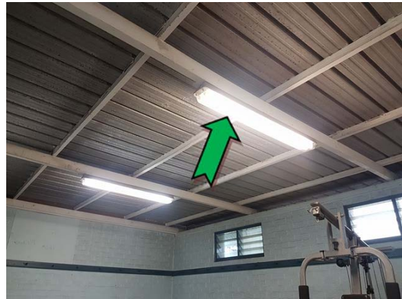
Photo 4. Interior, throughout, double tube fluorescent light fitting – suspected non PCB-containing capacitors.
