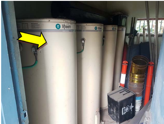
Photo 3. Interior, store room, hot water heaters – suspected SMF internal insulation material.
