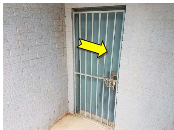
Photo 6. Exterior, throughout, doors – suspected lead-containing blue upper paint systems.
