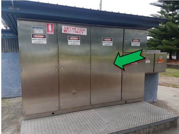
Photo 1. Exterior, north-east elevation, electrical backing board – suspected non asbestos-containing bituminous backing boards.
