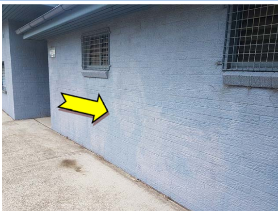
Photo 5. Exterior, throughout, walls – suspected lead-containing blue upper paint systems.
