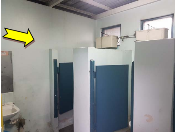
Photo 7. Interior, female and male toilets, walls – suspected lead-containing light blue upper paint systems.
